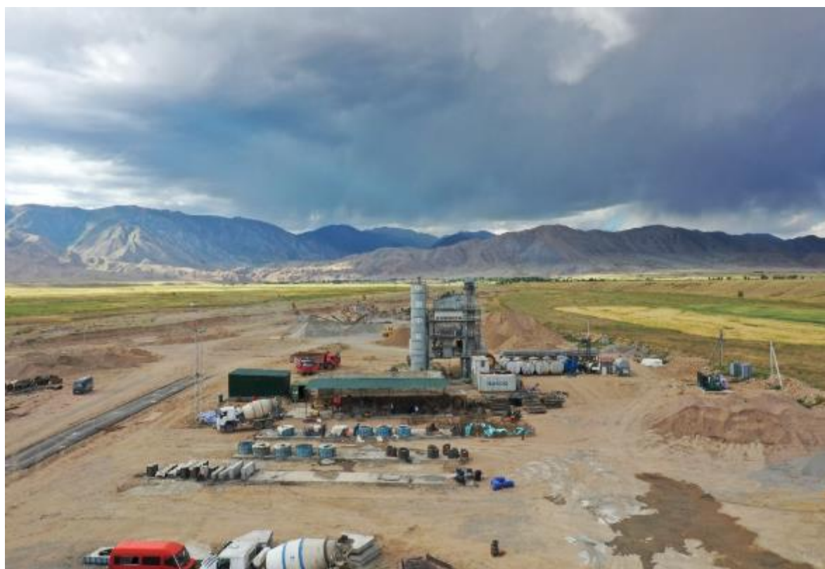
Figure 9: Asphalt plant at the production site (km 148+630)
